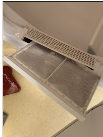
Clean out dryer vent on a yearly basis to prevent possible overheating/fire hazard.
