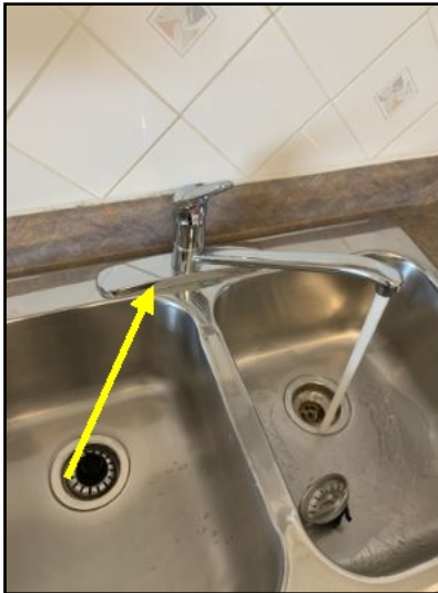
Loose faucet noted, repair required
