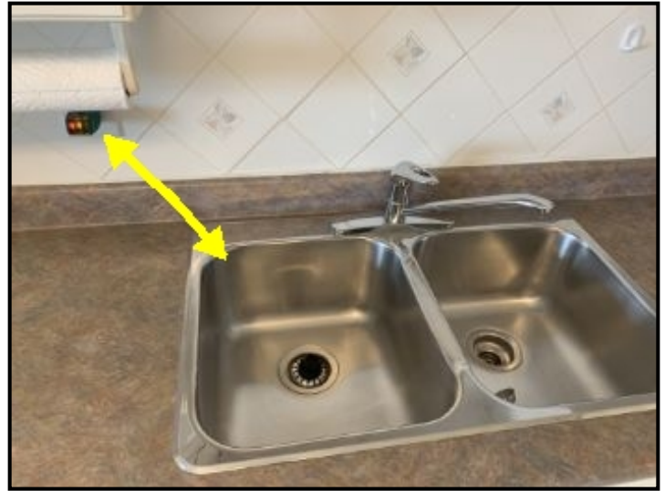
Note: GFCI outlets within 6' of sink are recommended for safety
