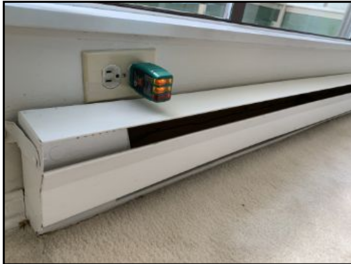
Receptacles placed dangerously close to baseboard heater, keep cords off and away to prevent melting/scorching
