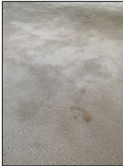
Stained flooring noted
