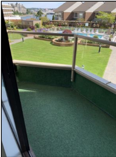
Have carpet removed from decks. (Causes rotting of wood planks.)
