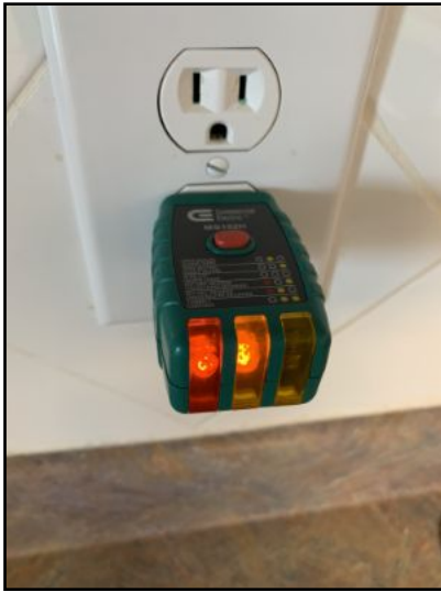
Reverse polarity or non-working outlets noted. Repair for safety
